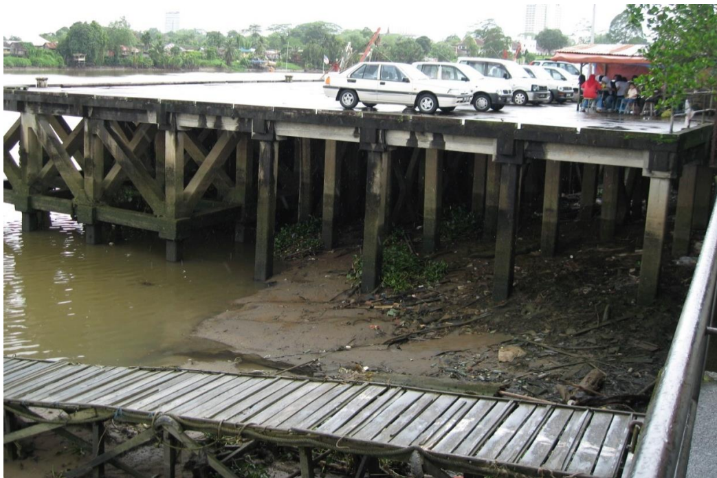
Figure 14 Ugly and dirty river banks during low tide. Survey of landing facility (SIWT UNDP 2008)
